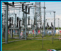
Power Station energy storage
