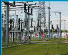
Power Station energy storage
