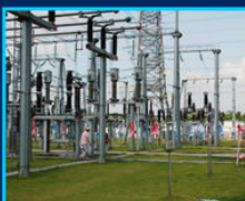
Power Station energy storage
